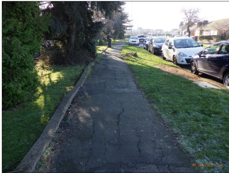
Figure 1 - Damage to footpath
