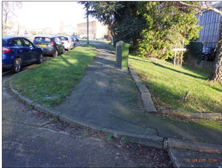
Figure 3 - Damage to footpath
