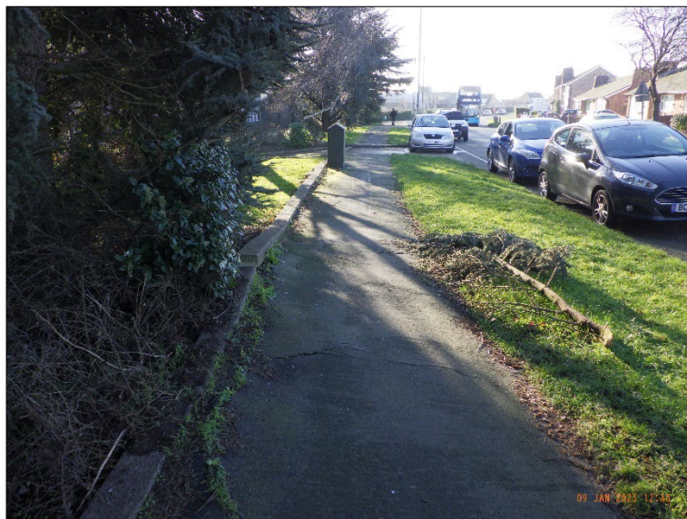
Figure 2 = Damage to footpath
