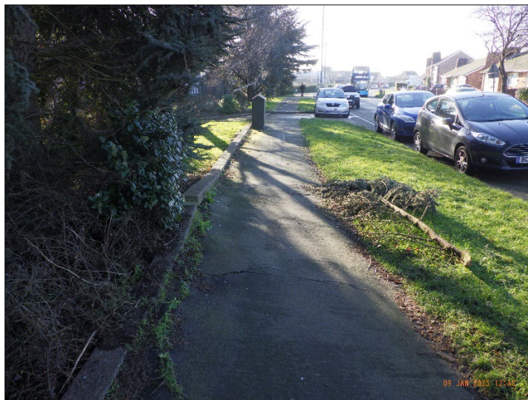
Figure 2 - Damage to footpath
