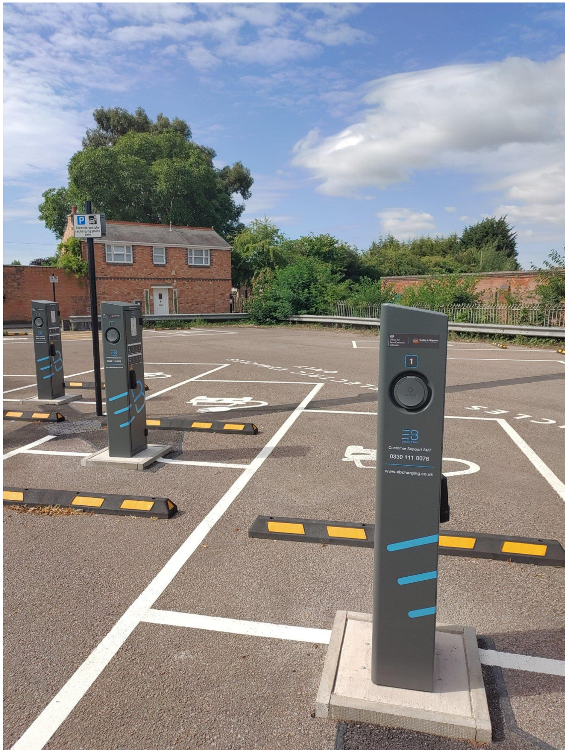
EV chargers in Countesthorpe Road car park, South Wigston
